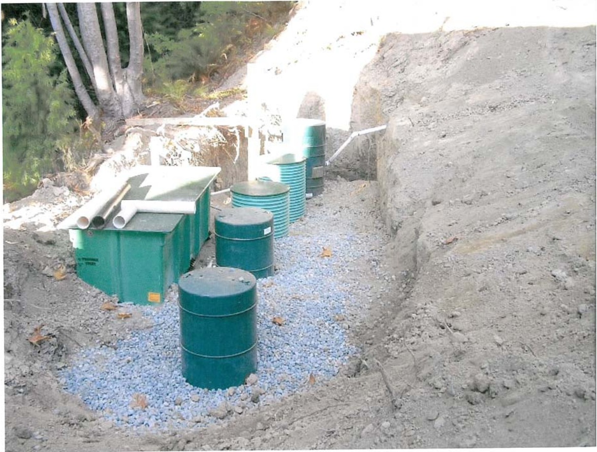
Image of Package Sewer Treatment Plant
